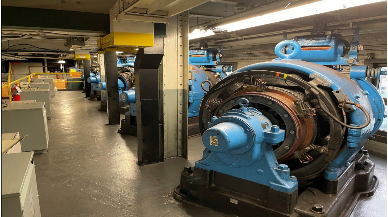
Photograph 11. Elevator penthouse motor level.
