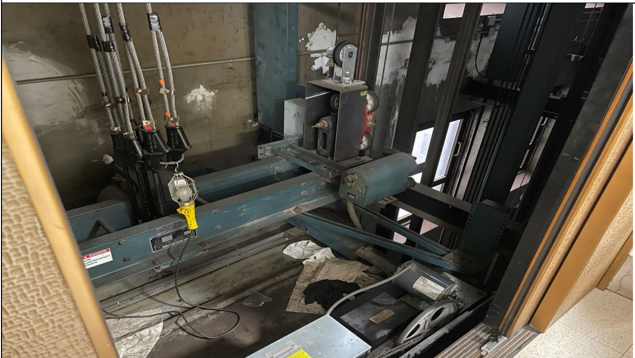
Photograph 6. Top of elevator car.
